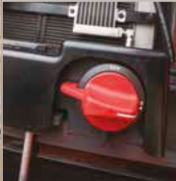
Battery cut-off switch
