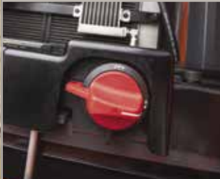
Battery cut-off switch
